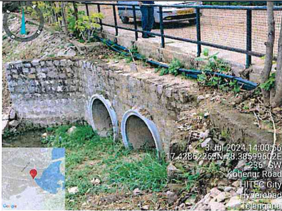
Durgam Cheruvu storm water drain inlets
