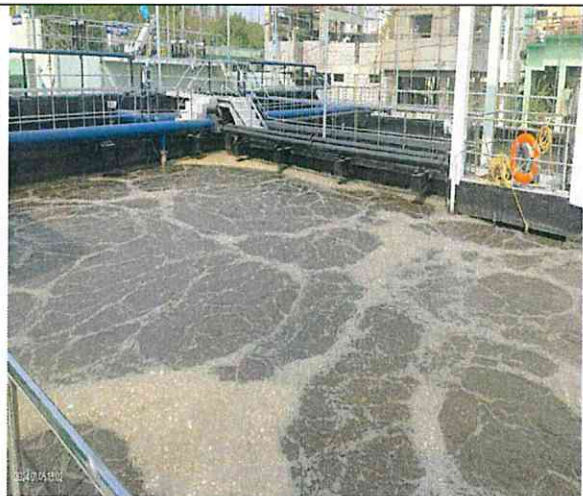
Durgam Cheruvu STP aeration tanks
