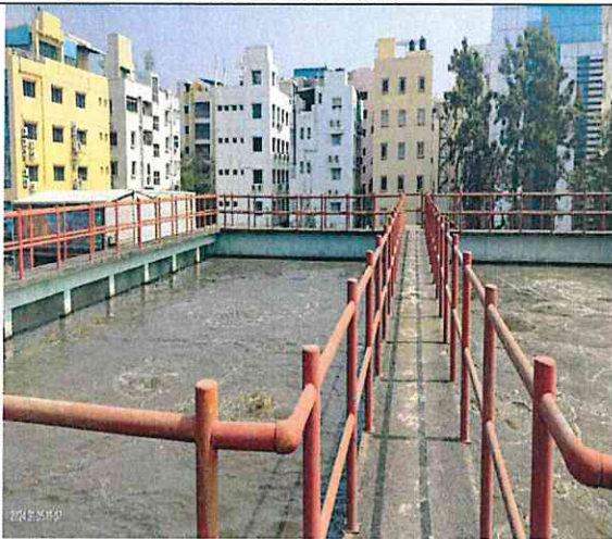
Durgam Cheruvu STP aeration tanks
